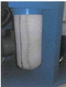
Cartridge Filter Location Inside Motor Cover
