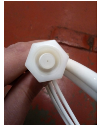
Another image of a flow restrictor in situ
